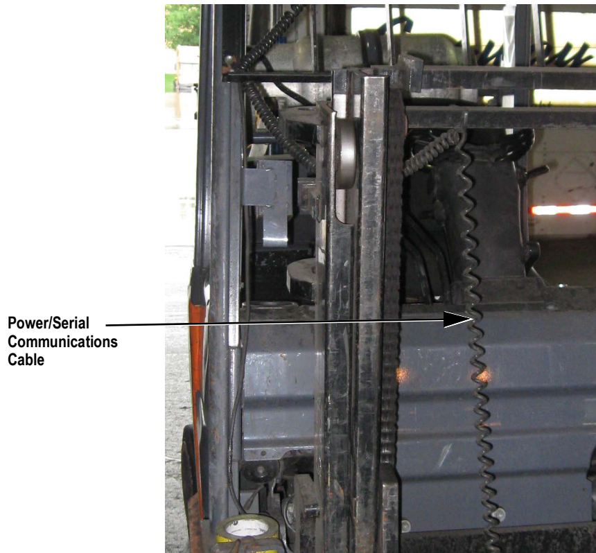
Figure 3-20. Signal Cable Located Between the Scale and the Indicator
